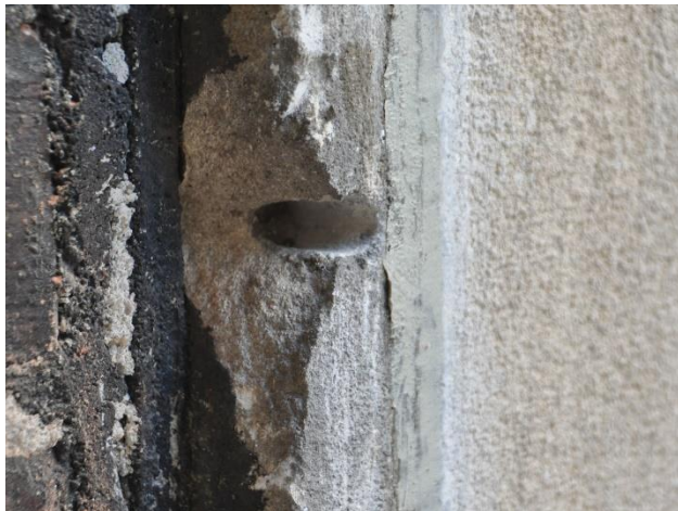
Figure 21 - Stone damage at the lead plug attachment.
