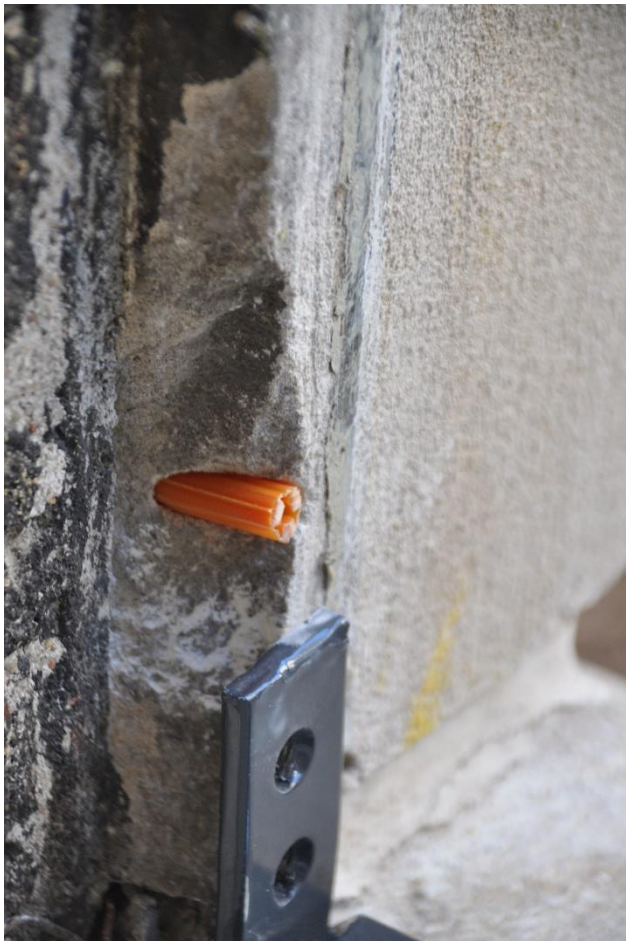
Figure 28 - A view of one of the plastic expansion shields in place in an area where the stone was damaged by the original expansion anchor.
