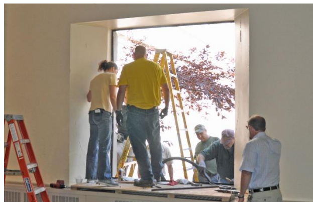
Figure 6 - The subframe is cleaned with an industrial vacuum cleaner so that the anchor attachments into the masonry wall can be found.
