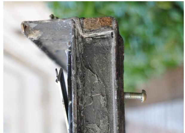
Figure 19 - View of the wood blocking at the window head reveals that the wood is in excellent condition.
