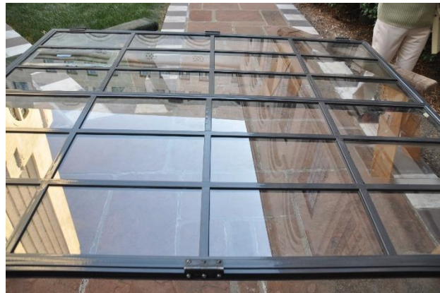
Figure 25 - The out of rack nature of the sash within the frames can be seen in the misalignment of the muntins.
