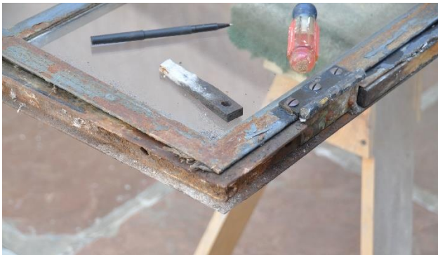
Figure 16 - After removal of the sash and frame assembly it was found that there was significant corrosion at the sill of the frame. However, the rest of the frame and the sash were in good condition.
