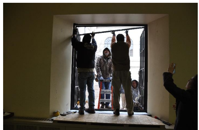
Figure 32 - The drip cap being installed between the subframe head and frame head.
