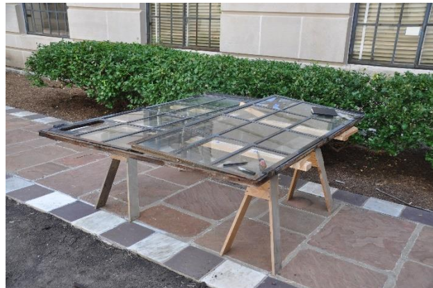
Figure 5 - The entire assembly composed of the frame into sash were removed in one piece.
