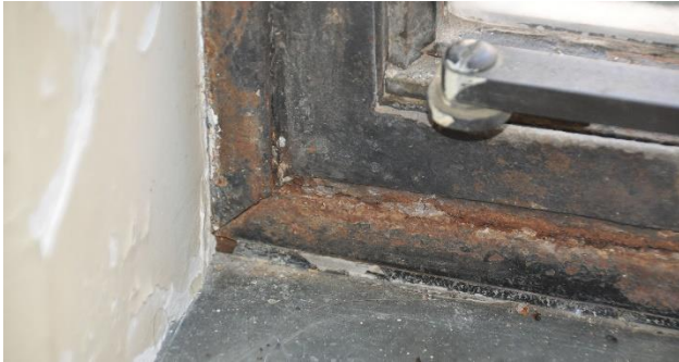
Figure 15 - View of the interface between the frame and subframe at the lower left corner and sill reveals extensive corrosion buildup.
