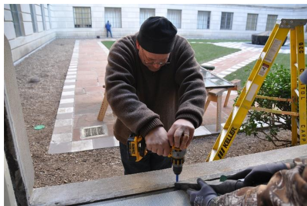
Figure 26 - The original holes in the stone were deepened to accommodate longer expansion anchors.
