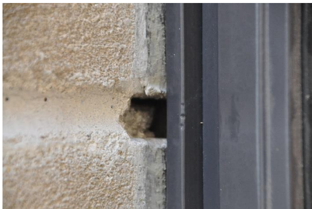
Figure 34 - The unfinished perimeter seal. This image shows that there will be some mortar work that will need to be implemented as part of the window restoration process.
