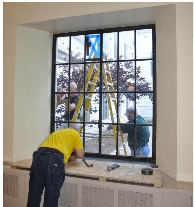
Figure 2 - The broken pane of glass has been taped so it will remain in place during the removal process. Workers on the outside are removing the perimeter sealant.
