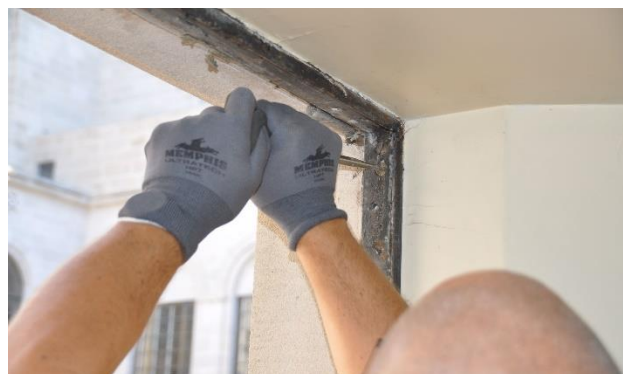
Figure 7 - The flathead countersunk metal screws attaching the subframe to the masonry beneath are removed by hand.
