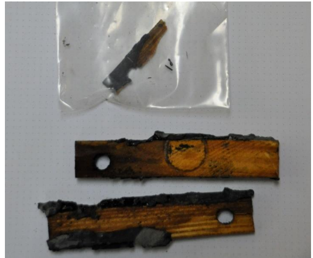
Figure 18 - Wood blocking removed from below the sill revealed the wood was severely damaged due to chronic moisture penetration.
