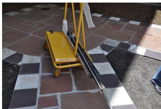
Figure 12 - The four subframe members have been catalogued and ready to transport to the shop.
