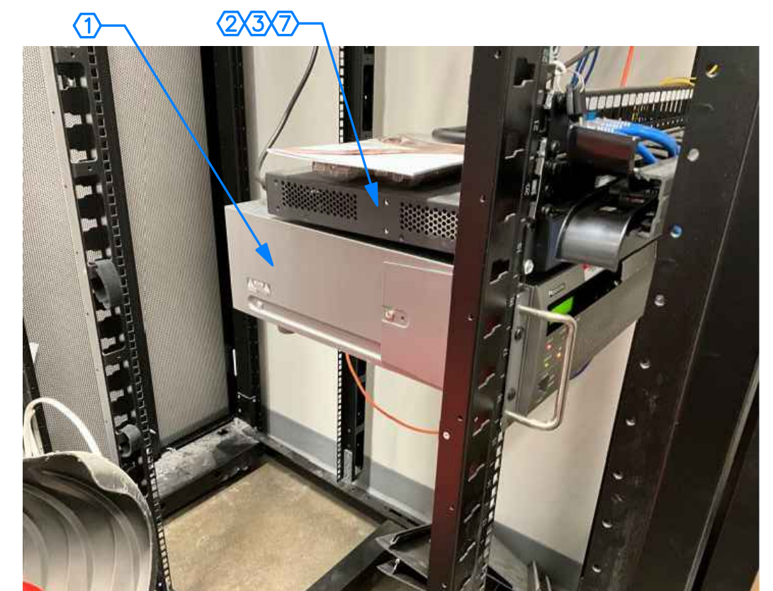
1C PHOTO EXISTING EQUIPMENT ES2.01 SCALE: NOT TO SCALE
